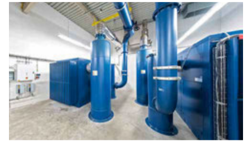
AERZEN screw compressors ensure perfect negative pressure at JTI in Trier.
