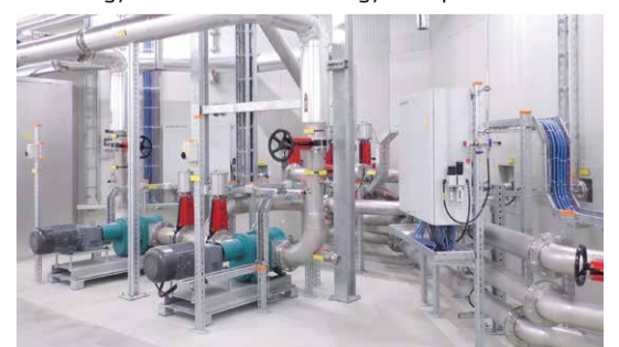
The Upper Engadine WWTP combines state-of-the-art technology with a sustainable energy concept.
