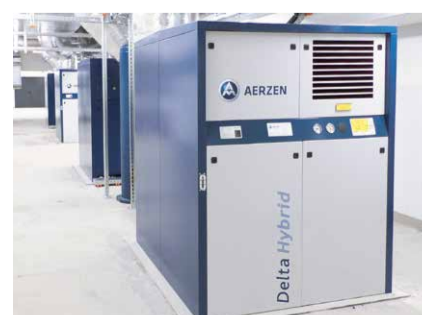
AERZEN Delta Hybrid D 52S rotary lobe compressors ensure optimum oxygen supply to the five SBR reactors.
